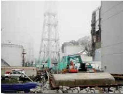
Three AVANTech employees traveled to Japan after last year's earthquake and tsunami to set up a water treatment system that removes radioactive isotopes.
